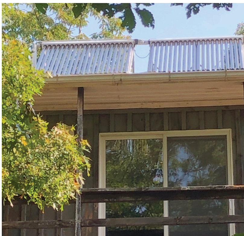
Top: Dederick's geothermal system, which he estimates cut his heating costs in half after he switched from an oil-fired furnace. Bottom: Evacuated tube collectors convert sunlight into photovoltaic energy.
